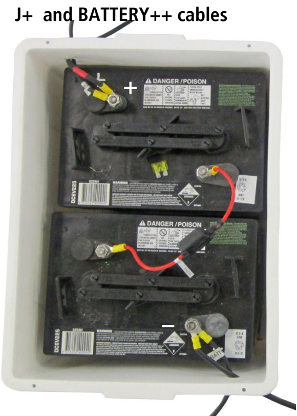
J+ and BATTERY++ cables
